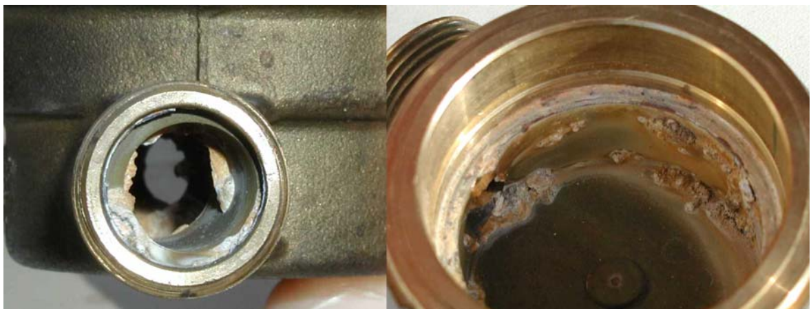
Figure 4. Limescale built-up in the inside of a single jet water meter housing
